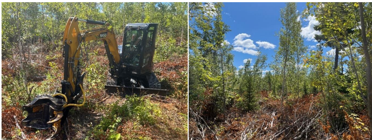
Figure 8. Excavator with a shear head conducting a mechanical pre-commercial thinning operation in North Forks, New Brunswick
