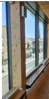
Radiant hydronic systems located under most windows.
