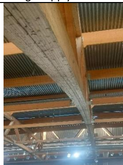
The large laminated wood lattice girders.
