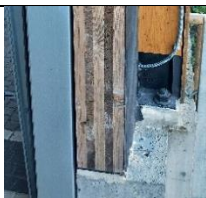
Evidence of weathering at the CLT edge-grain
