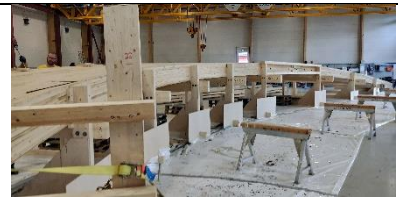
Double curvature bridge with creosote and CCA treatment, 10mm bitumen & 50mm of asphalt for 100+ year life.
