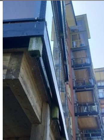
Untreated timber balconies.
