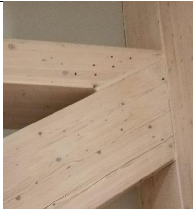
Glulam columns as large as 0.6 m by 1.5 m were used in the structure.
