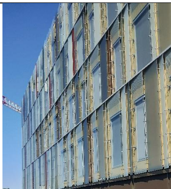
Triple glazing curtainwall windows with automated operable fabric shading elements.
