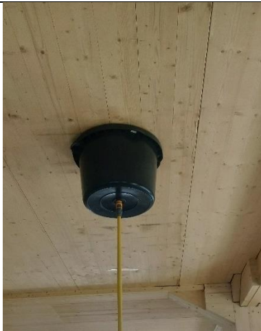
Drain piped externally for each CLT bay
