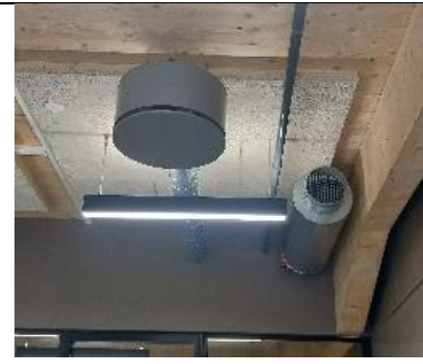
Ventilation ducts visible in the ceiling.
