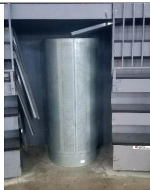
Large supply air ducts.
