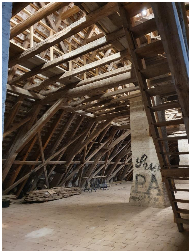
Figure 8 Skokloster Castle was started in 1656. The massive roof structure has been painstakingly restored using traditional techniques.
