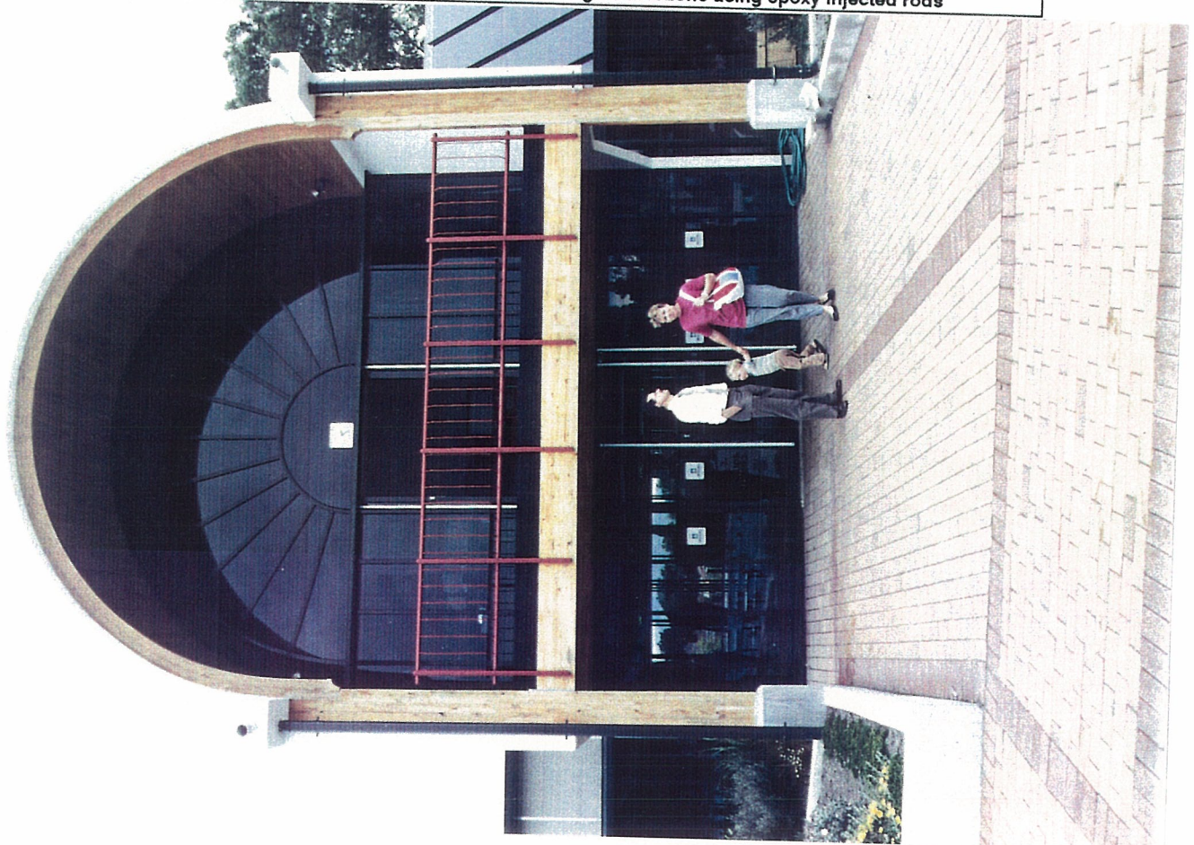
Photograph 2.10 - Entry to Jelly Park Pool - moment resisting connections using epoxy injected rods
