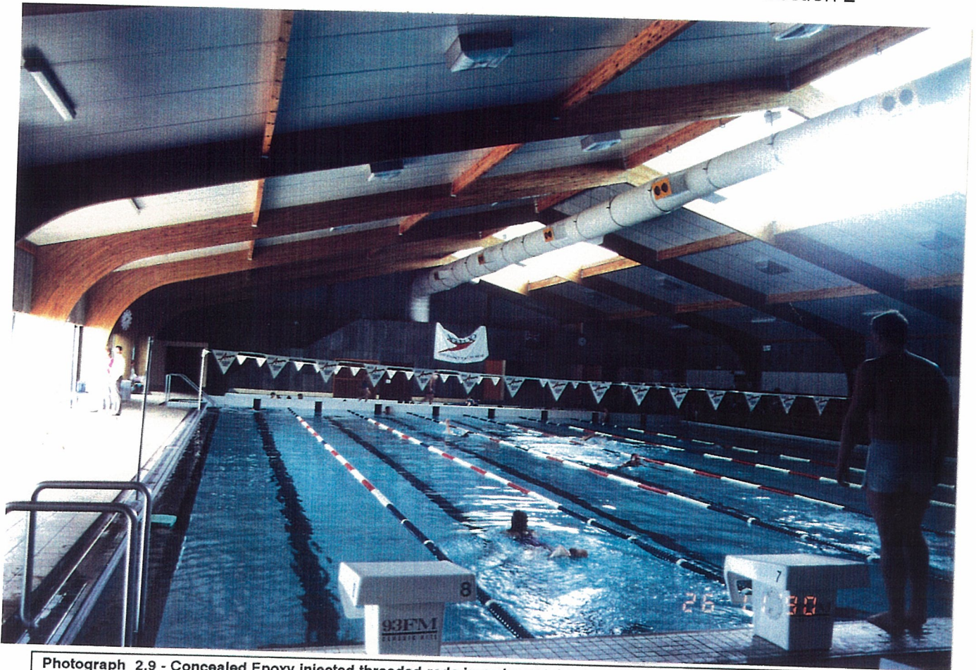
Photograph 2.9 - Concealed Epoxy injected threaded rods in main portal arches for indoor pool enclosure at Jelly Park Pool, Christchurch NZ
