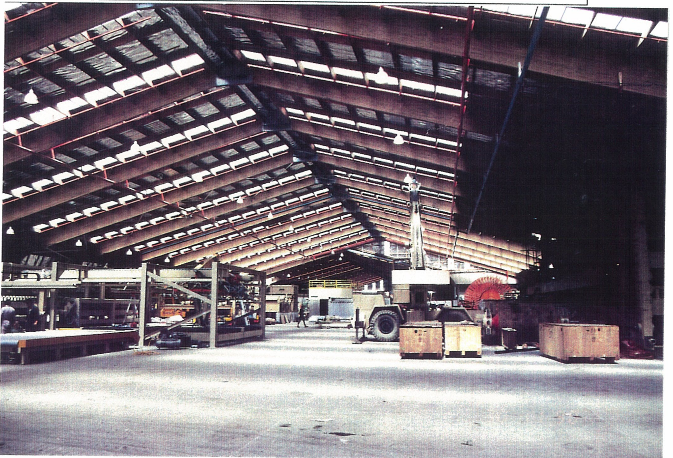
Photograph 4.2 - An example of glulam construction - 56m clear span MDF factory - Nelson NZ Timber supplied by Hunter Timbers, Nelson
