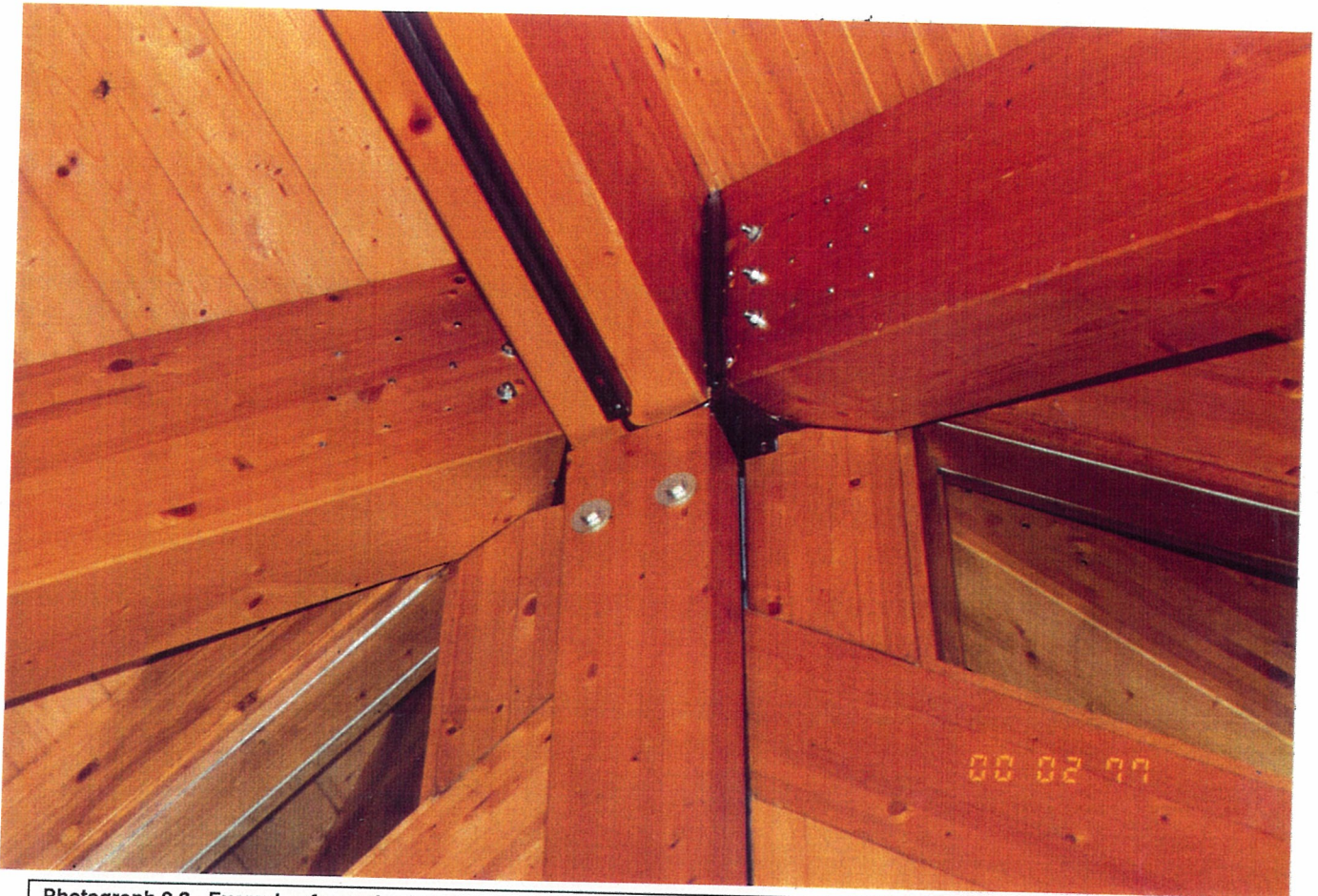
Photograph 2.3 - Example of complex Fin-plate dowelled connection. Church at Gucy - (near Lausanne, Switz)
