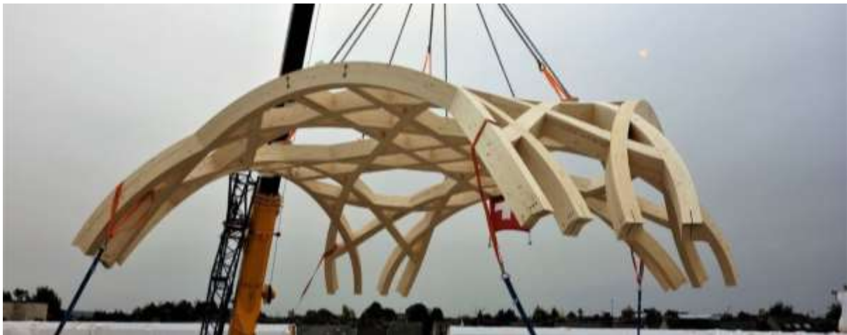
Figure 72 Figure 72 Roof component of the Cambridge Mosque by Marks Barfield Architects and Blumer Lehmann Photo: https://i2-prod.cambridge-news.co.uk/incoming/article14033374.ece/ALTERNATES/s1200/Mosque-1.jpg
